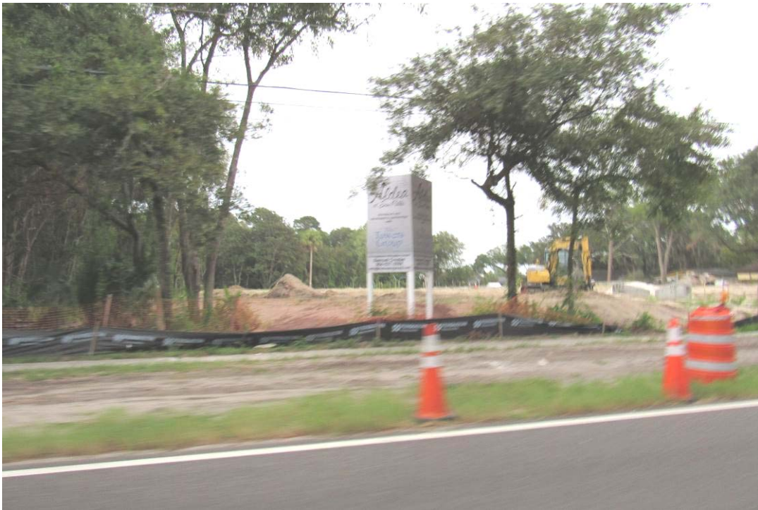
Subdivision under construction across San Pablo Road. It is complying with the minimum standards in the RLD-60 Zoning District.
